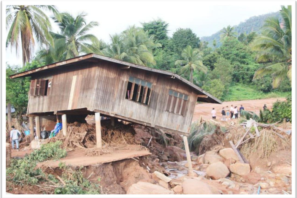
Photo 6: Cooperative members' House affected by the Flood (13 th Sept. 2011)
